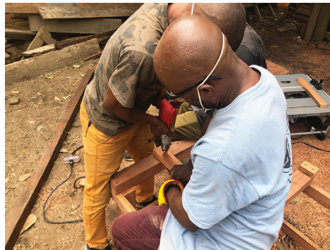
Two men work together to prepare a work bench to mount the new table saw and portable planer supplied to the carpentry training center
